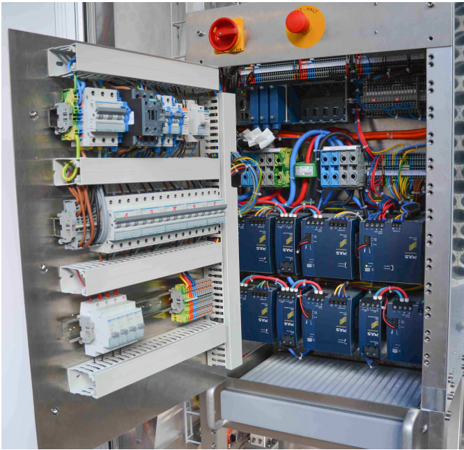
FIG. 6.5 – The safety control cabinet with circuit breakers for the 230 VAC safety and 3x400 VAC physics power and the redundant 24 VDC power supplies. The cRIO control system is installed at the top left side.
